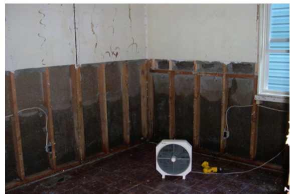
Drywall and insulation were removed immediately after the floodwaters receded in an attempt to minimize the damage. This home, like so many along Parkview Drive, was damaged beyond 40% of its Fair Market Value and determined to be Substantially Damaged.
