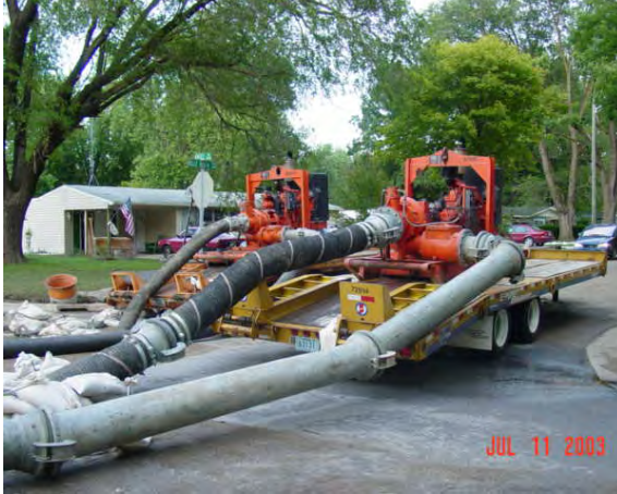
Huge pumps were brought into the Belle Vista neighborhood and Fernwood Drive area to pump floodwater from the streets and storm sewers back into the Fairfield Ditch.
