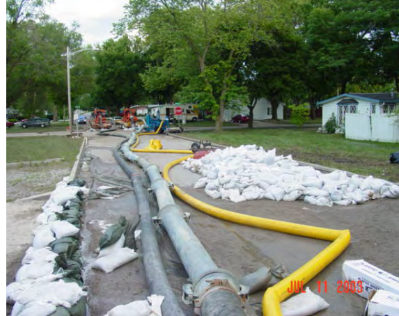
Hundreds of feet of pipe and conduit line the street to carry floodwater backing up in storm drains away from homes and discharged it back into the Fairfield Ditch.
